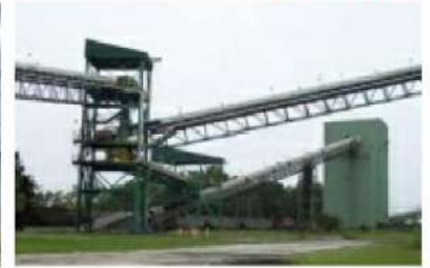
Power Plant Conveyor
